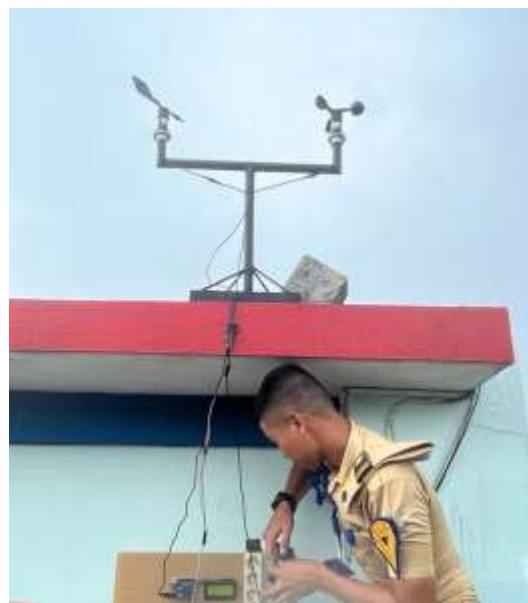
Figure 4. Test of the Wind Direction Indicator Display
