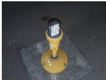
Gambar 3. Lampu Runway Bandara Sultan Thaha- Jambi
